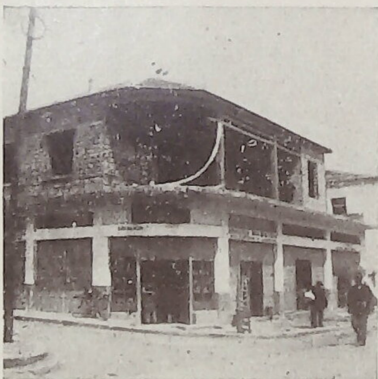
Fig. 7.—Failure of concrete joist arch due to improper location in the brick wall of a new building resting on thick, watersaturated alluvium in Pharsala during the earthquake of April 30, 1954.
