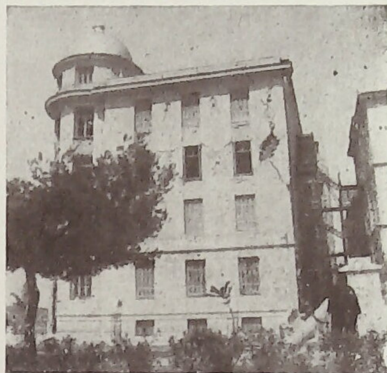
Fig. 6.—Damage to the east side of a well built five-story building resting on manmade fill near the quay of Volos during the earthquake of April 30, 1954. See in the foreground the memorial column thrown down.
